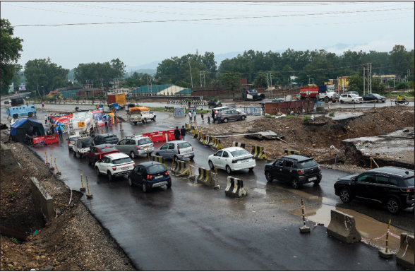
of the damage caused by the flash floods and landslides. In another incident, flash
